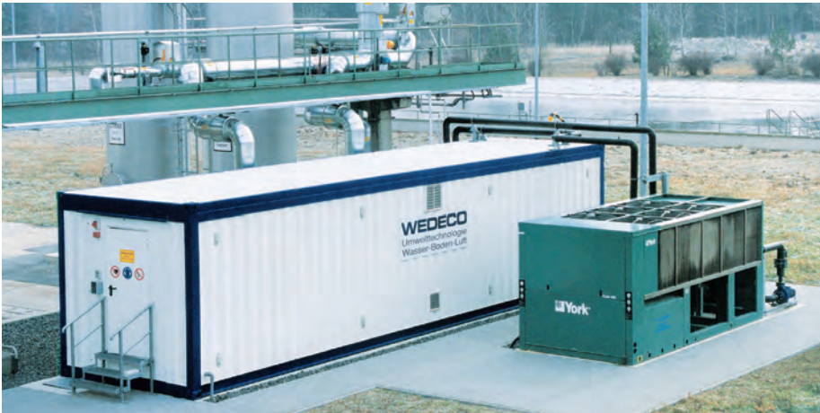
Ozone Generator with an Oxygen Plant and Chiller System
