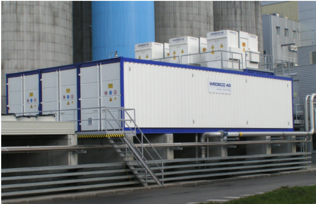
A CONTAINERISED OZONE SYSTEM IN A PULP MILL
