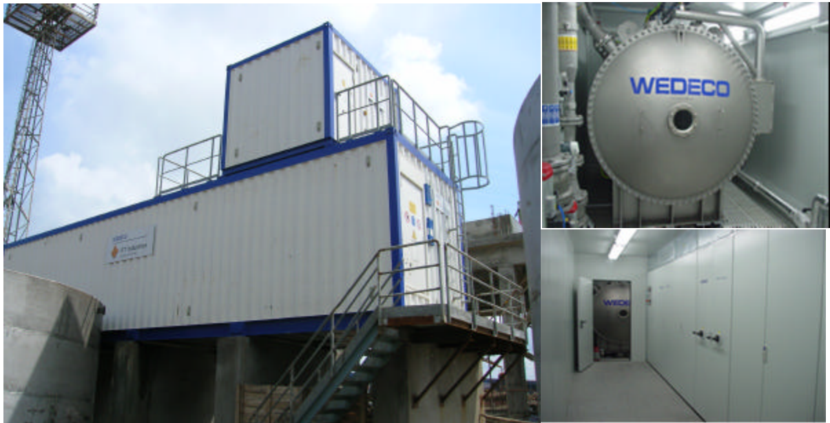
Figure: Worldwide largest single containerized Ozone Generator / ITC pulp mill.
